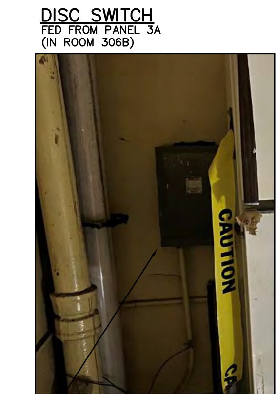
DISC SWITCH FED FROM PANEL 3A (IN ROOM 306B) NEW FEEDER FOR PANEL 3A SHALL ENTER THROUGH WALL OPENING AFTER THE REMOVAL OF DISC SWITCH.
